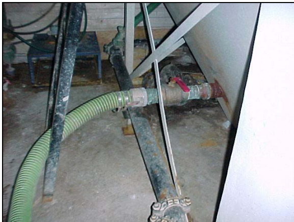
Photo 53 FTC clarifier manual dump valve & waste line.
