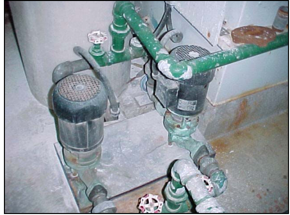
Photo 15 Freeze protection – recirculation system.
