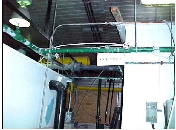
Photo 38 Raw water pipe to FTC unit.
