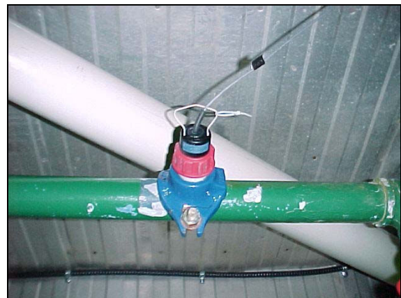
Photo 9 Paddlewheel flowmeter – raw water.
