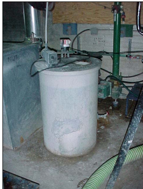
Photo 50 Polymer chemical system for FTC .
