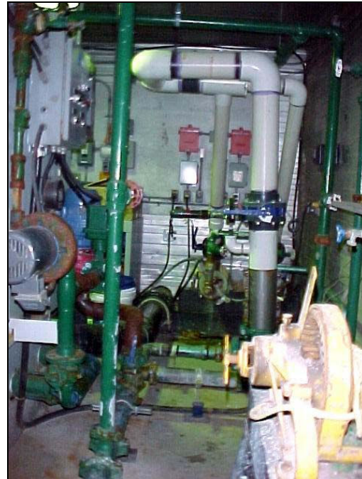
Photo 3 Raw water intakes @ water plant.
