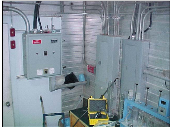
Photo 33 Auto transfer switch for the genset.
