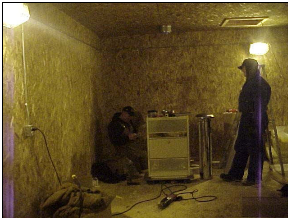
Photo 79 Interior lights & drip furnace.
