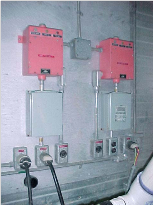
Photo 28 Heat trace controllers.
