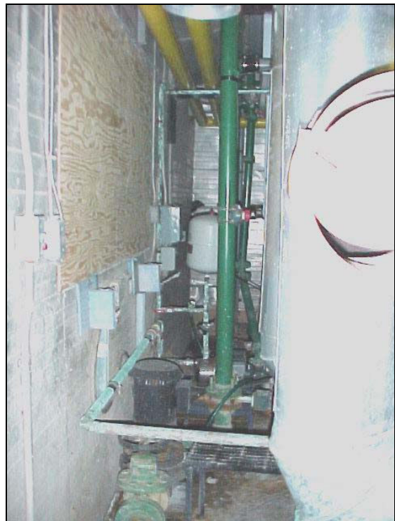
Photo 17 Truckfill pump and pipe c/w flow sensor.
