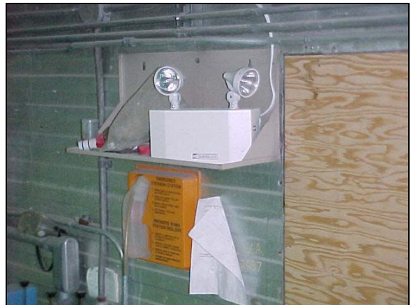
Photo 83 Eyewash station & emergency light..
