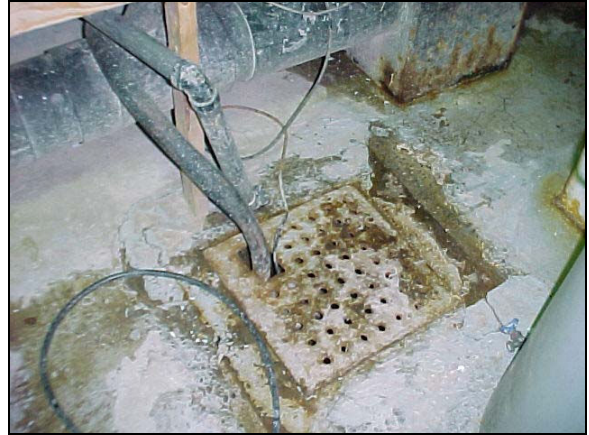
Photo 56 Building waste sump.
