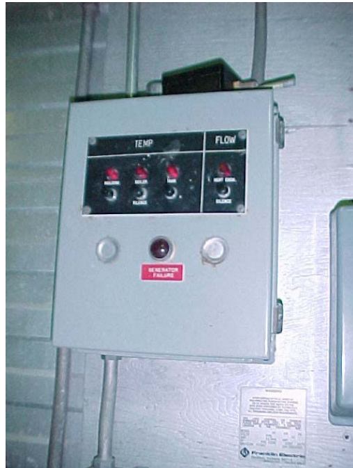
Photo 61 Main alarm panel inside WTP.
