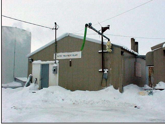
Photo 90 Truckfill with rigid hose prior to modifications.
