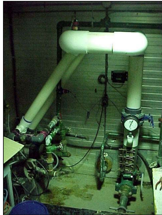
Photo 13 Intake backwash system.
