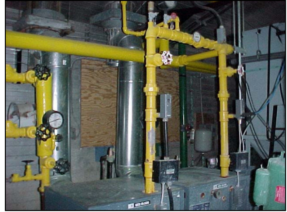
Photo 23 Boiler system with process pipings.
