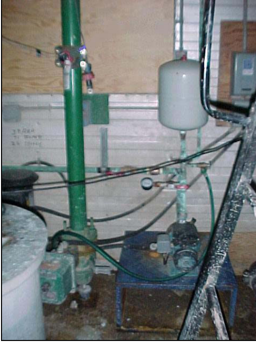
Photo 18 Domestic cold water system.
