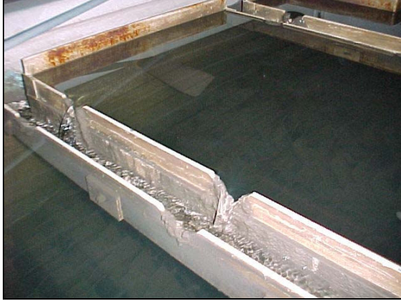
Photo 37 Clarifier in the FTC unit.
