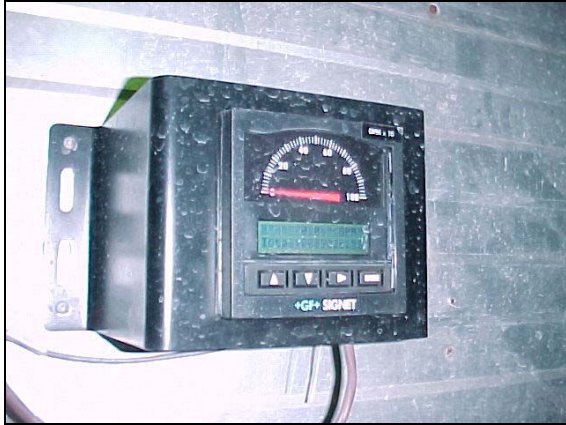
Photo 10 Flow/totalizer meter – truckfill system.
