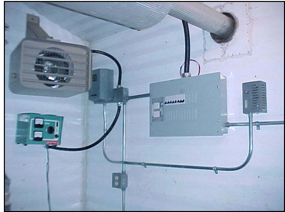
Photo 65 Electric heater for building heat, electrical sub-panel and thermostat.
