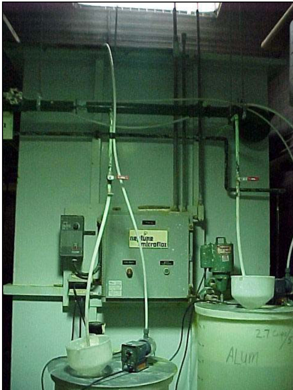
Photo 35 FTC control panel & chemical injection point.
