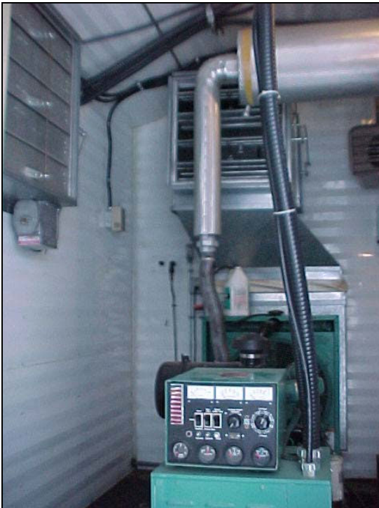
Photo 68 Genset engine exhaust.
