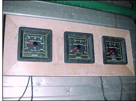
Photo 11 Flow totalizer meter – raw water
