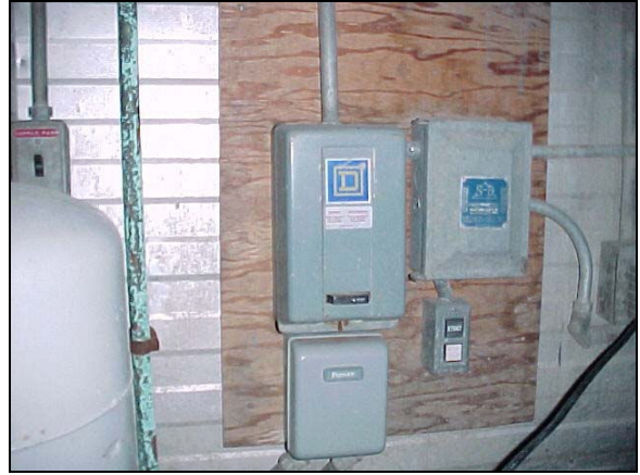
Photo 31 Truckfill pump motor control panel
