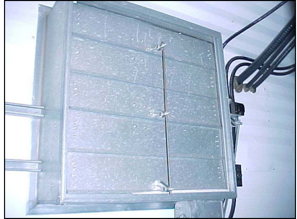
Photo 67 Fresh air intake.
