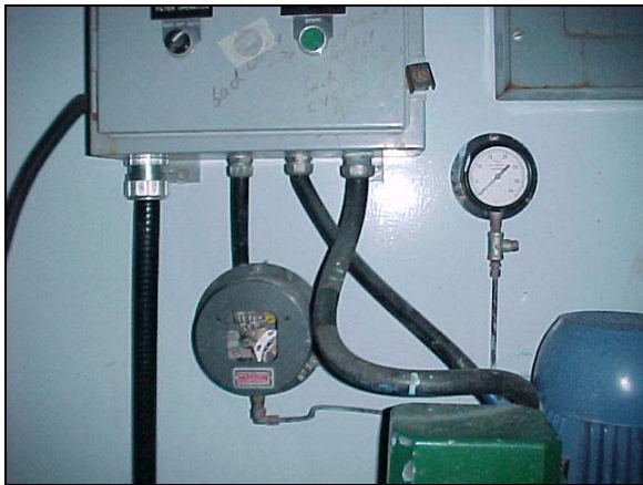
Photo 45 Headloss gauge below the Control panel.
