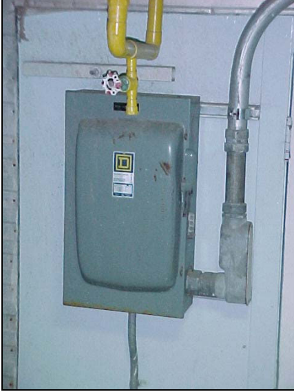
Photo 26 Main disconnect @ water plant.
