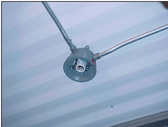
Photo 72 Missing light bulb.
