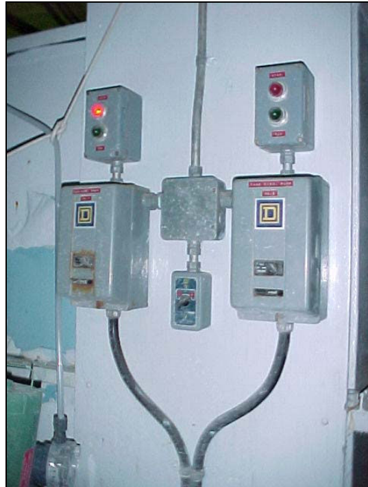
Photo 29 Recirculation pump motor panels – freeze protection
