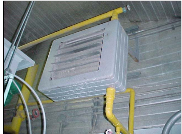
Photo 21 Unit heater – water plant.
