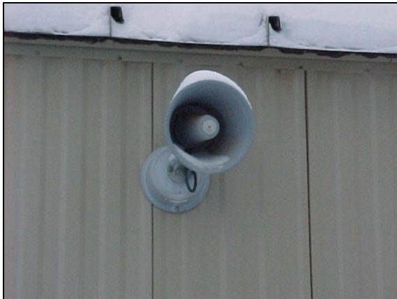
Photo 60 Audio alarm outside WTP.
