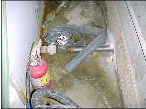
Photo 55 FTC flocculation chamber drain line to outside of WTP..
