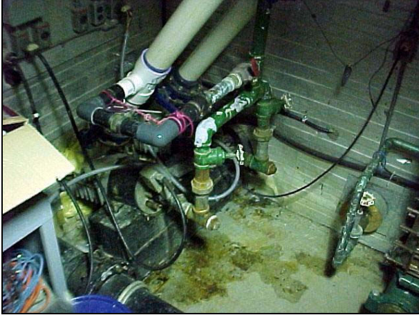
Photo 4 Raw water intake @ water plant.
