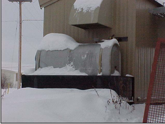
Photo 74 Fuel tank & cooling air exhaust for genset building.
