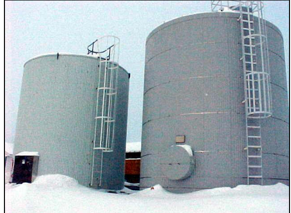
Photo 59 New storage tanks.
