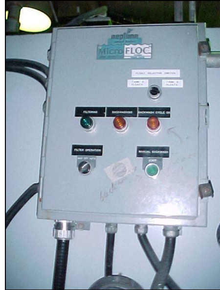
Photo 44 WTP control panel.
