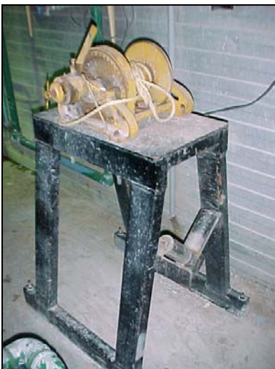
Photo 8 Winch for pulling intake pumps.
