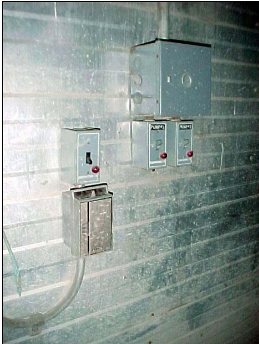
Photo 32 Thermostat & boiler recirculation pump switches
