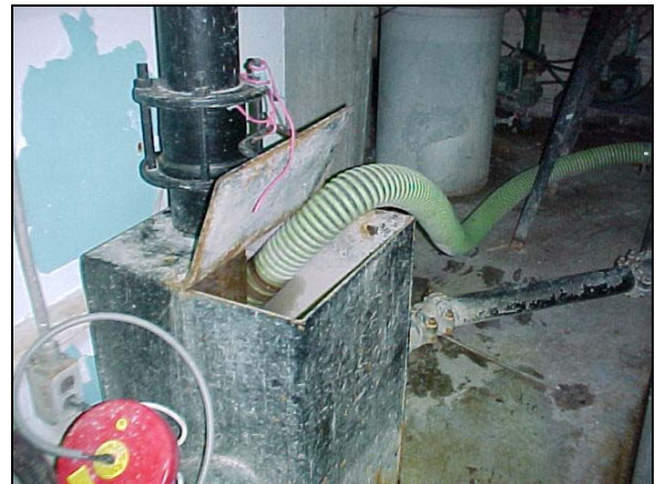
Photo 54 Waste line from FTC clarifier to waste disposal system..
