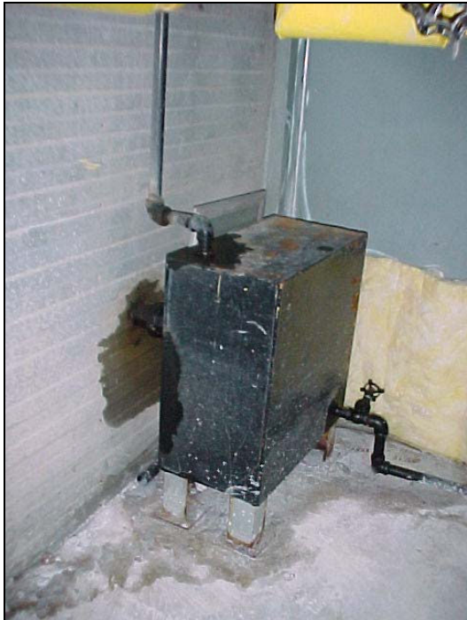
Photo 24 Day tank for the boiler system.
