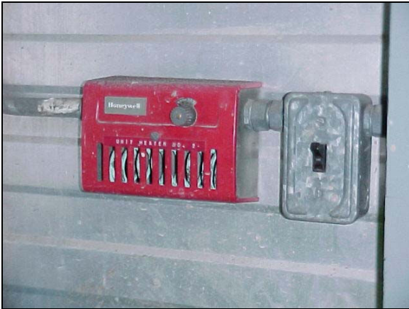
Photo 20 Low temperature alarm – water plant.
