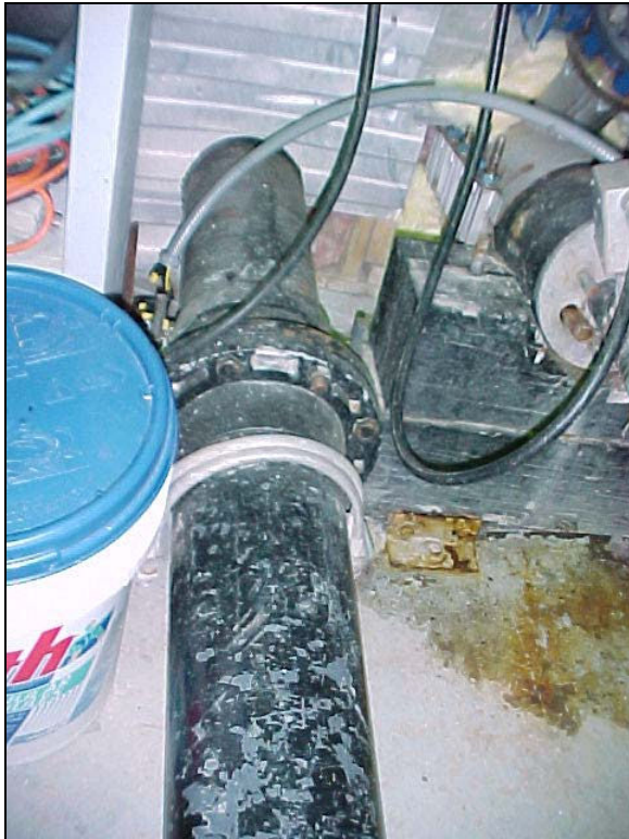
Photo 57 HDPE waste line to Peel River.
