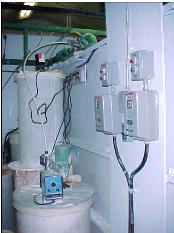
Photo 49 Powdered chlorine feed system @ Waterboy.
