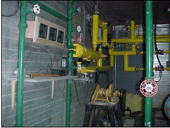
Photo 14 Heat tempering system - process pipings.
