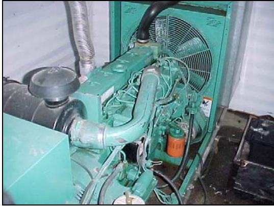
Photo 70 Genset engine and battery.
