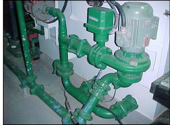
Photo 48 Waterboy backwash pump.
