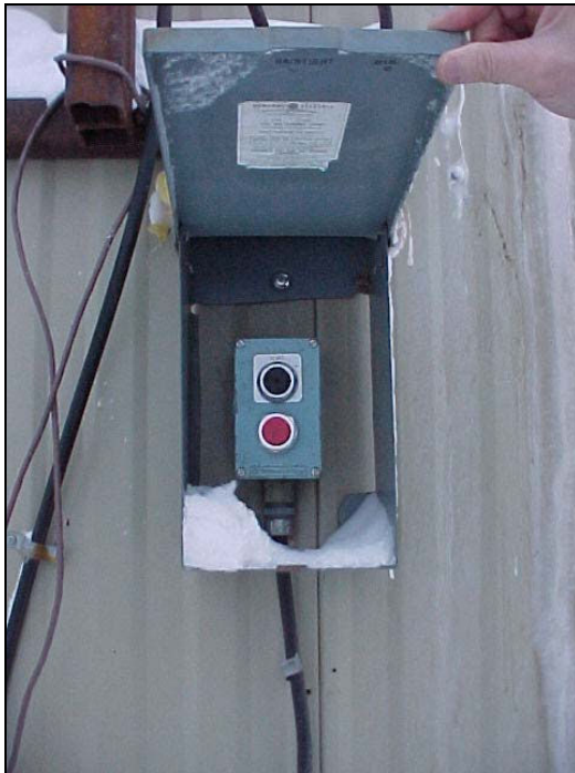
Photo 88 Outside truckfill panel.
