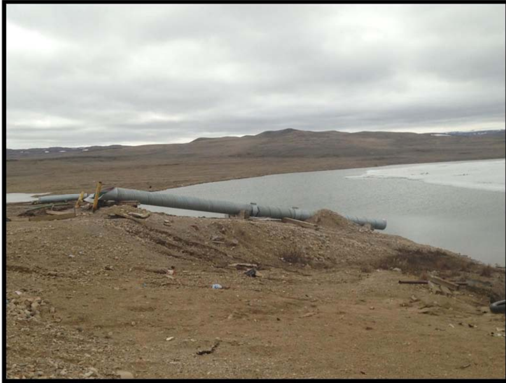
Figure 13: Sewage Discharge Pipe into the Sewage Lagoon
