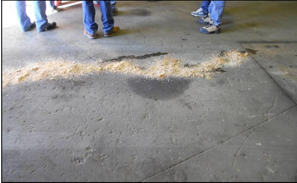
Figure 3.3: Absorbent Material placed over Spilled Vehicle Fluids
