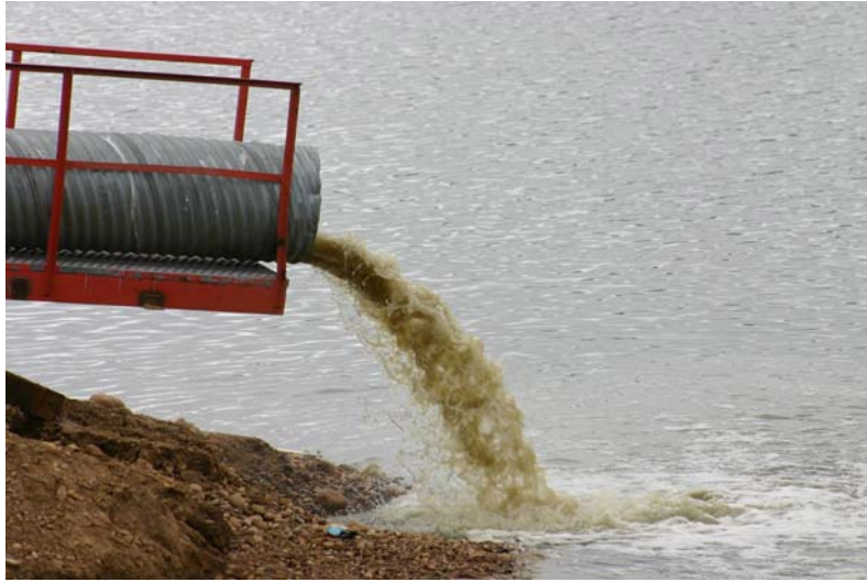
Figure 3 - Discharge of Sewage to Lagoon
