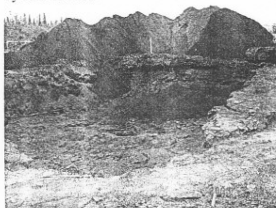
Figure 4. Excavated contaminated area showing aerated soil in background. The soil is to be placed back in excavated area by Alu bucket.
