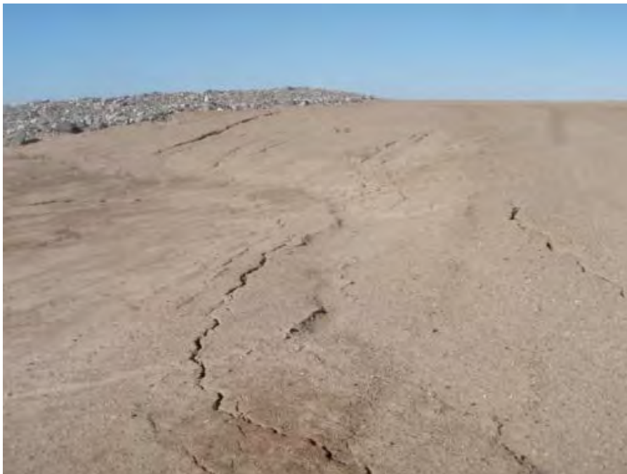
Photograph 10 – Signs of settlement on the east side of Landfill A (Section 3.1.7).
