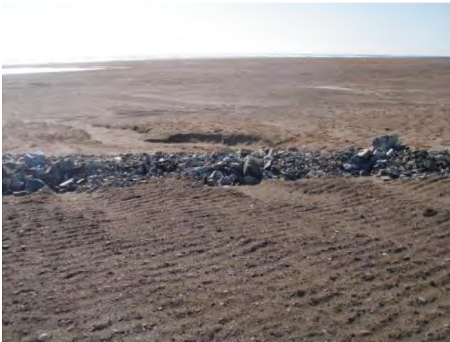
Photograph 13 – Signs of erosion near the southwest corner of Landfill A, looking toward the Prince of Wales Strait. A seasonal drainage channel is evident downslope (Section 3.1.7).
