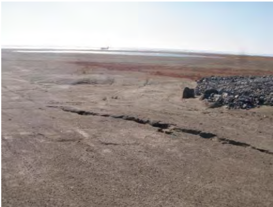
Photograph 11 – Erosion channel on the east side of Landfill A, up-slope from the settlement (Section 3.1.7).
