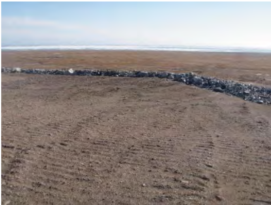
Photograph 19 – Landfill D – The 2010 report indicated that water was ponded in this area on the cap (Section 3.1.10).
