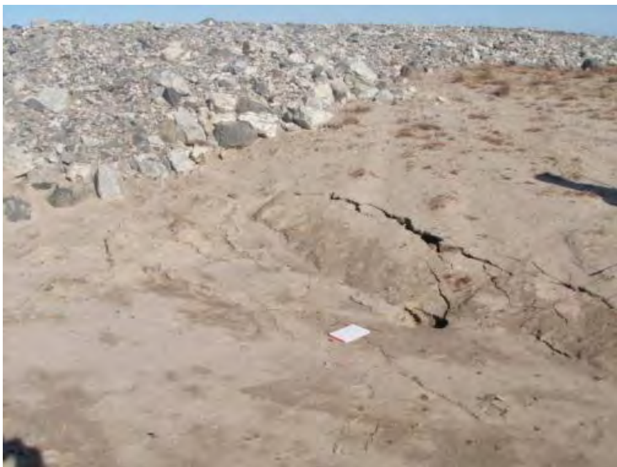
Photograph 12 – Erosion channel on the south side of Landfill A (Section 3.1.7).
