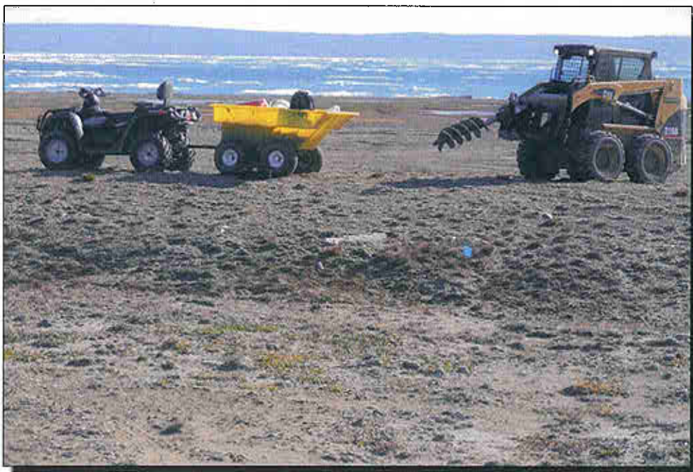
Photo 4 Area B, Lobe E, note surface debris.
