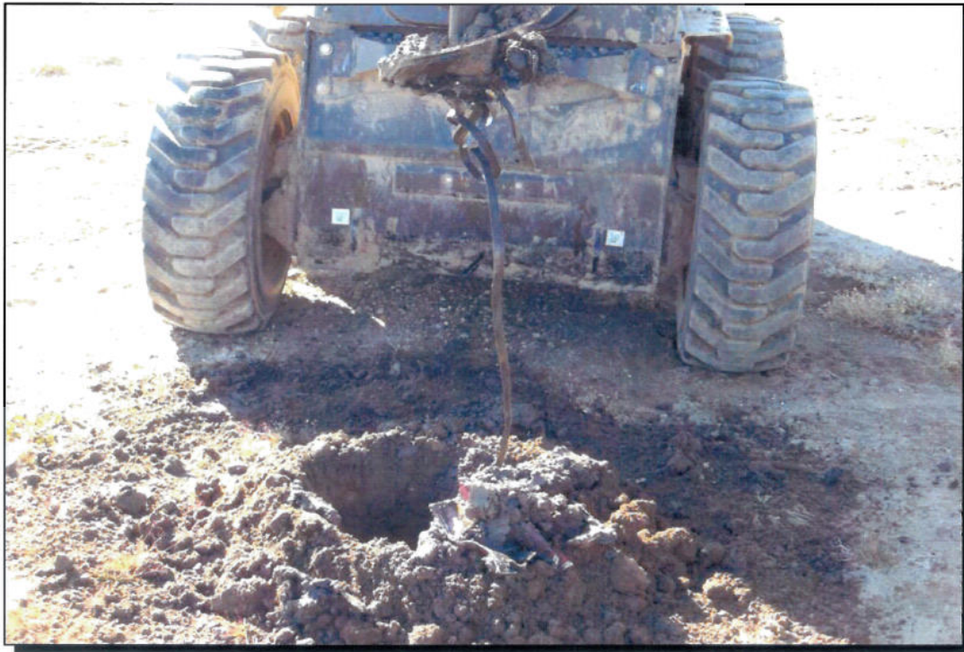
Photo 19 Existing Landfill A – metal debris from landfill
