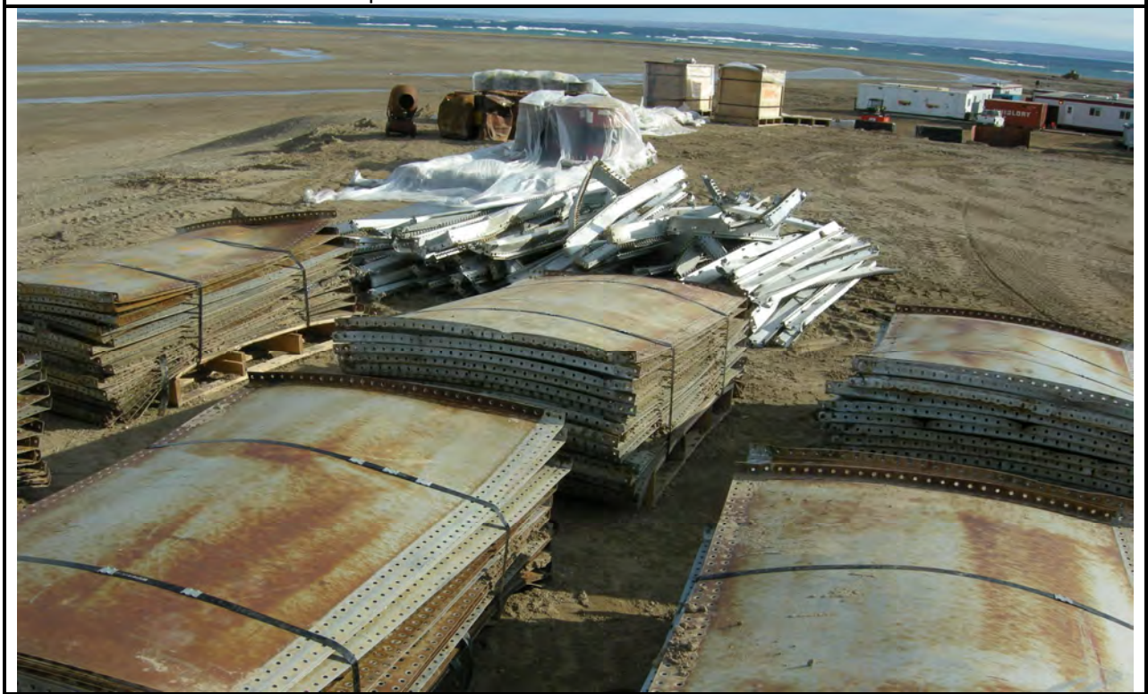
Photo 22: Palletised POL tank sections
