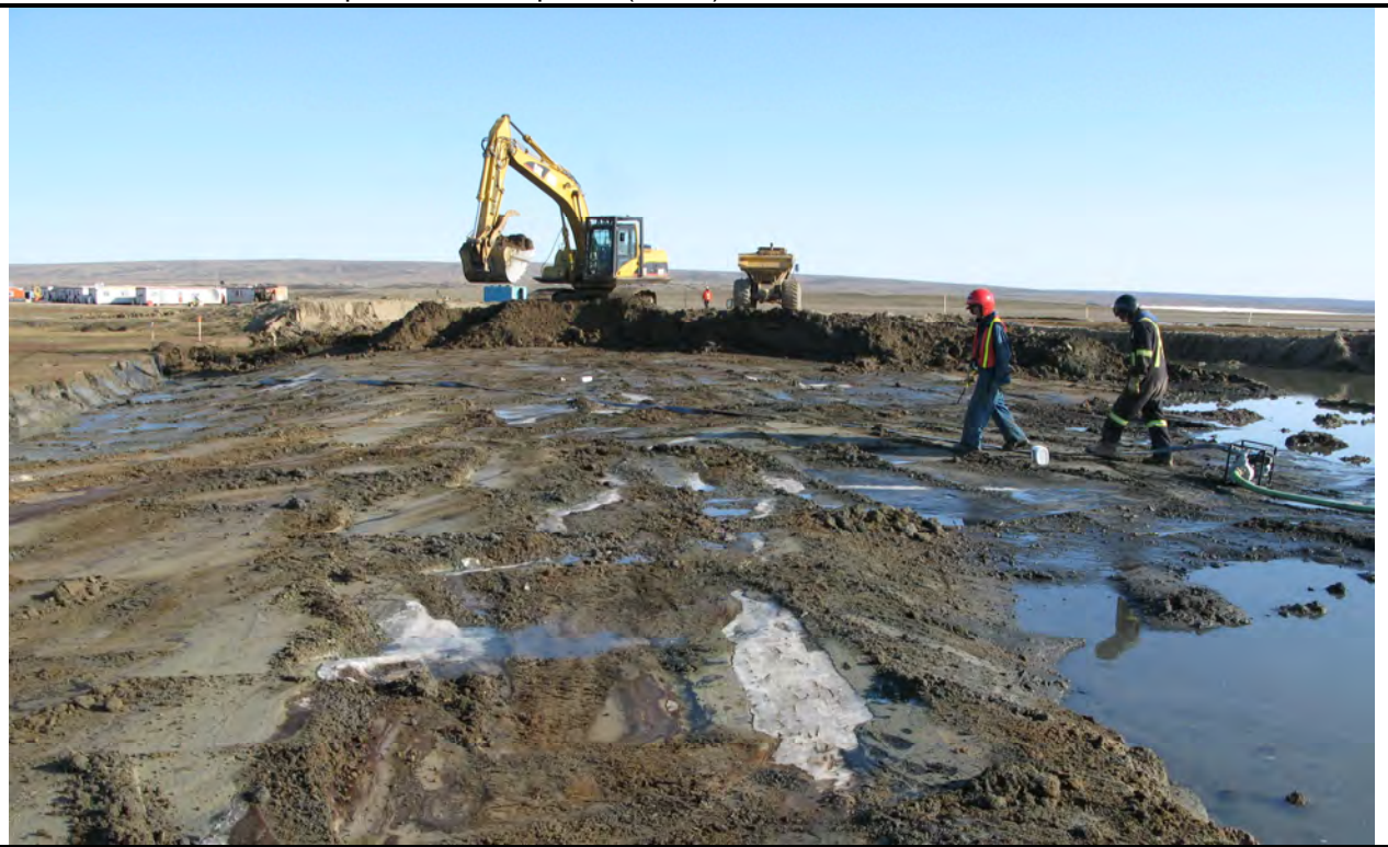
Photo 30: Excavation of Apron Area SW plume (Part 1). Note ice lens at base of excavation
