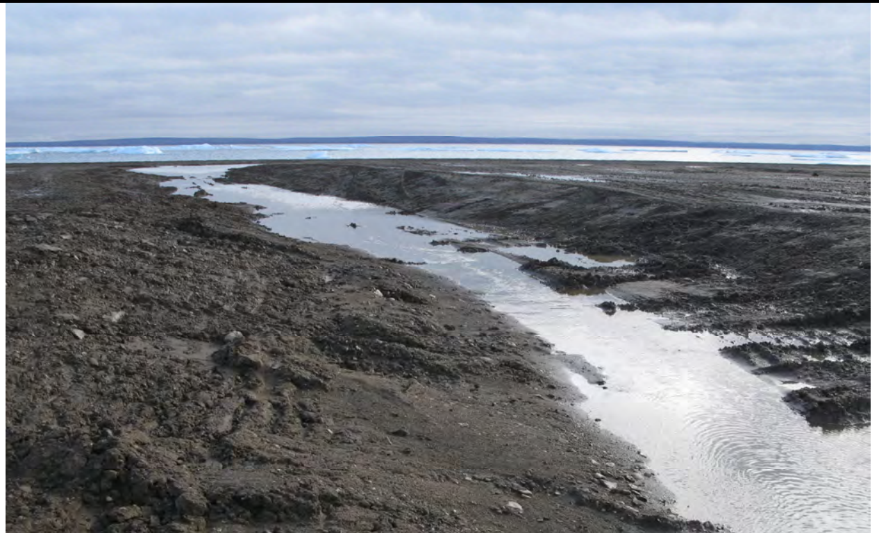
Photo 42: Swale at south end of the Airstrip following removal of culvert at the close of the 2009 season
