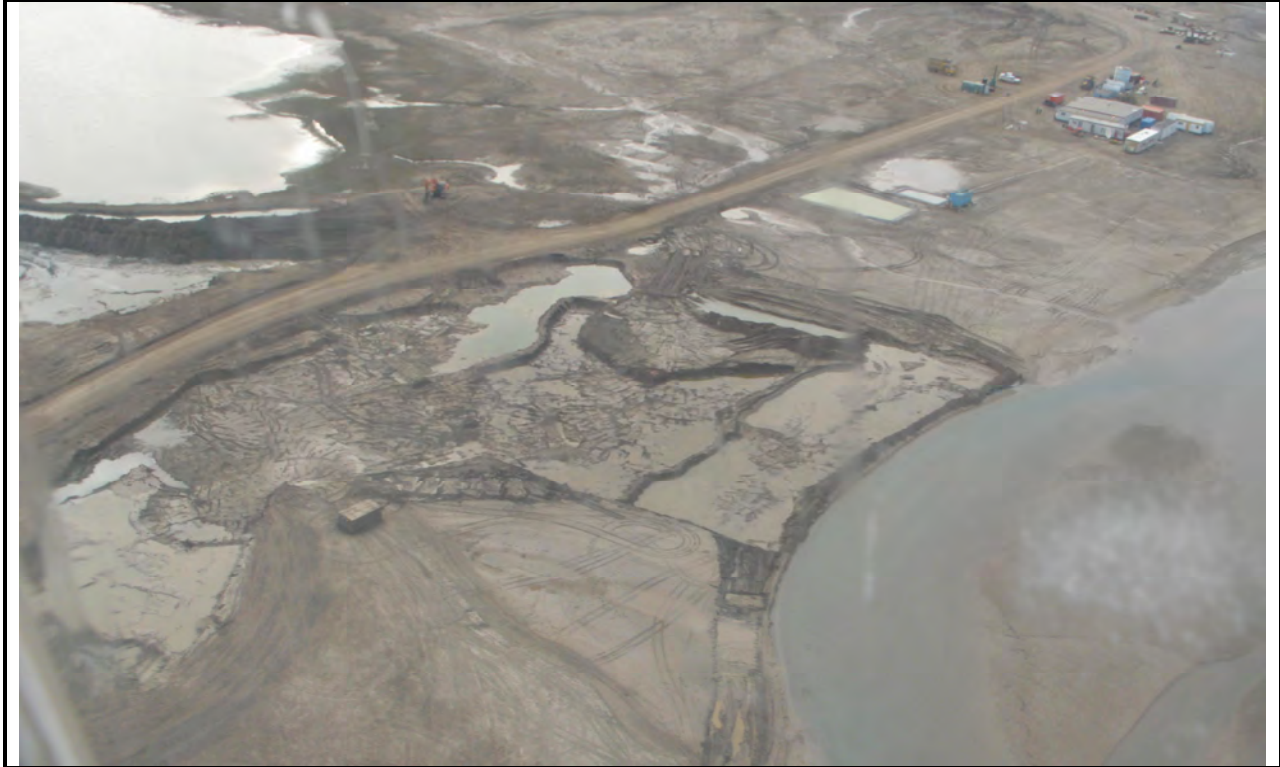
Photo 5: View of Apron area excavation with construction camp in top right corner and greywater treatment system between camp and excavation
