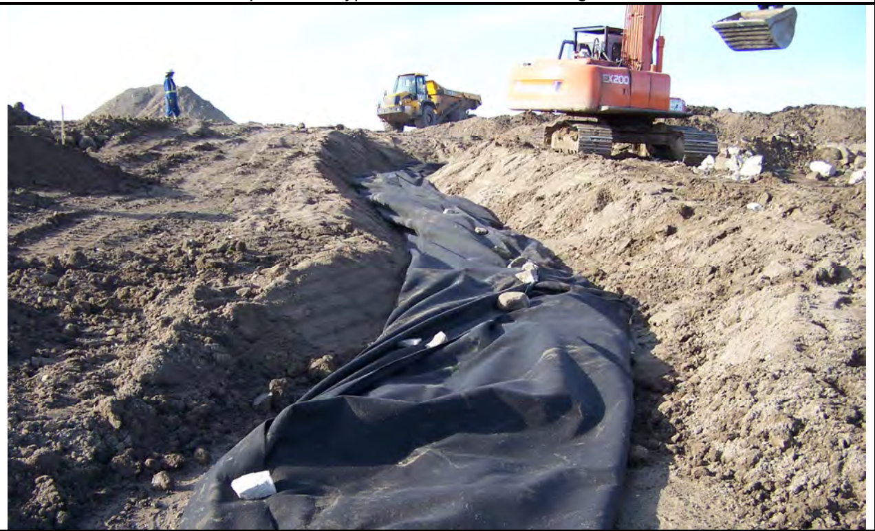
Photo 34: Type 1 Material and geotextile French Drains along base of Landfill Regrade A
