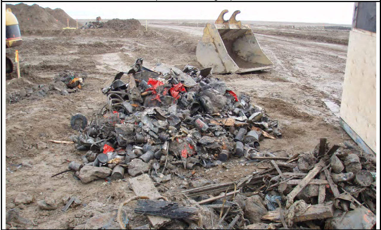
Photo 28: Debris removed from Buried Debris Lobe P
