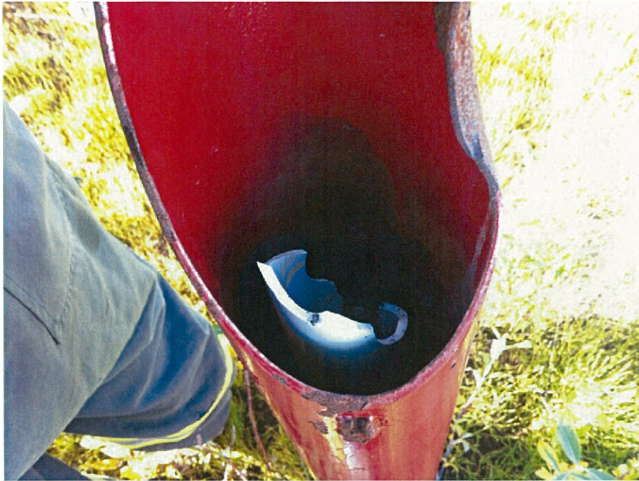
Photograph 1: View of damaged monitoring well MW 1 (September 2, 2013).
