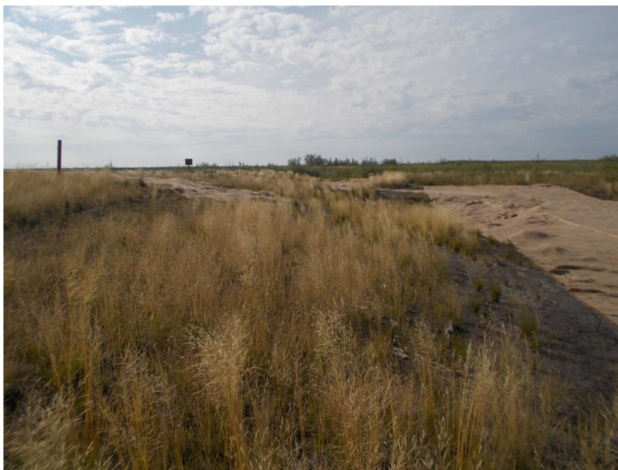
Photograph 9: Coconut matting staked down over area of sparse vegetation on western and northern portion of backfill cap (August 12, 2014).
