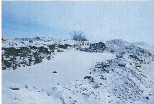
Figure 1 Flare pit excavation filled in with water from the adjacent river. The surface area was bermed so as to avoid flooding the ice.
