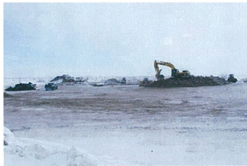
Figure 3 Lined storage area for the excavated contaminated material from the sump has been removed.
