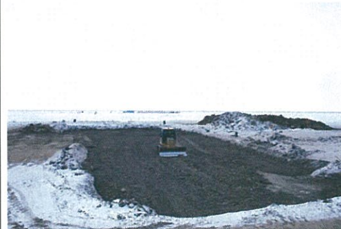
Figure 4 Excavation is almost fully backfilled. Can barely see the outline of where the excavation was located. Overburden and material from the sandbar borrow source is put down in lifts then compacted with a packer and watered down.
