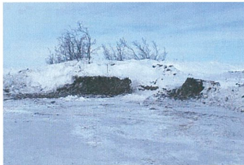
Figure 5 Camp sump excavation has been backfilled and restored to match the surrounding bank.
