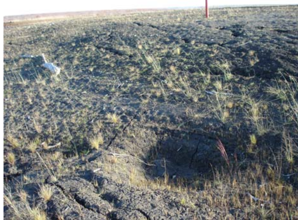
Figure 4 Sink hole at the sump excavation. Continued monitoring is needed to assess any further subsidence and to mitigate possible risks to site stability, October 2, 2012.
