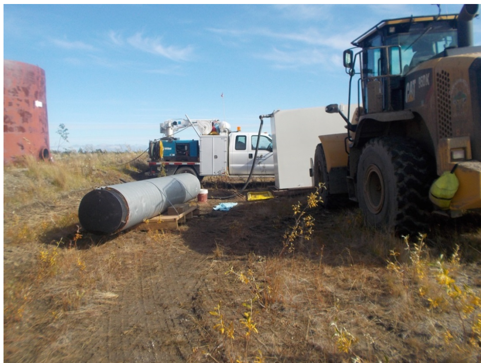
Photograph 13: Transferring contents of large tank in tank farm to small portable tank (August 17, 2014).
