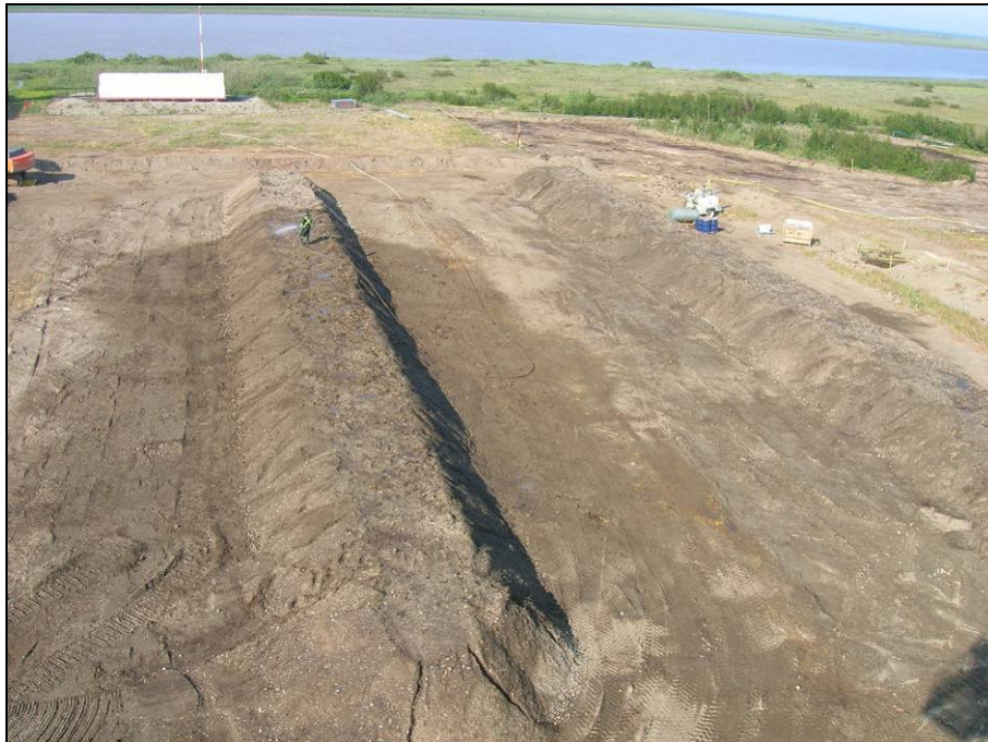
Photograph 4: North end of Camp Farewell treatment cell, water is being applied to windrow 2. Excavation 1, the largest area of excavation is visible in the right background.
