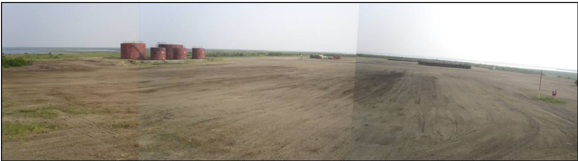
Photograph 10: Panorama looking northeast from camp building. Portion of backfilled excavation #1 at left and regraded treatment cell area in centre.
