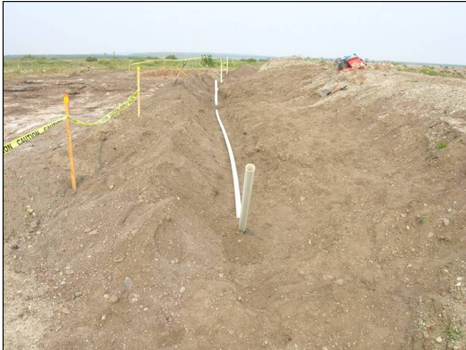
Photograph 6: In situ subsurface treatment trench and 50 mm piping system prior to backfilling looking north. Tank farm berm at right, excavation #1 at left.
