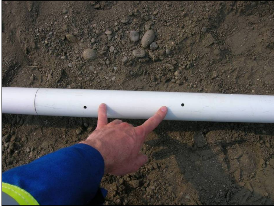
Photograph 7: Perforations made on-site. Holes are spaced around all sides of the pipe.
