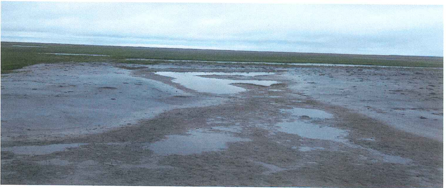
Figure 5 Water Ponding on sump, July 21, 2020
