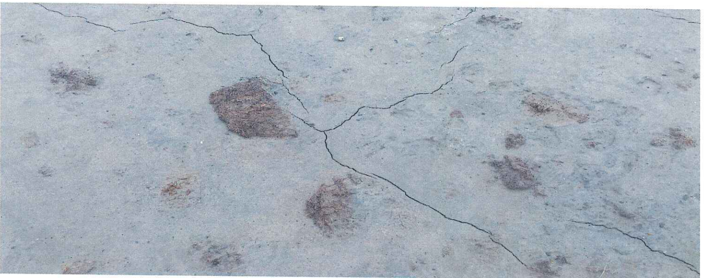
Figure 3 Cracking on sump new cap, July 21, 2020
