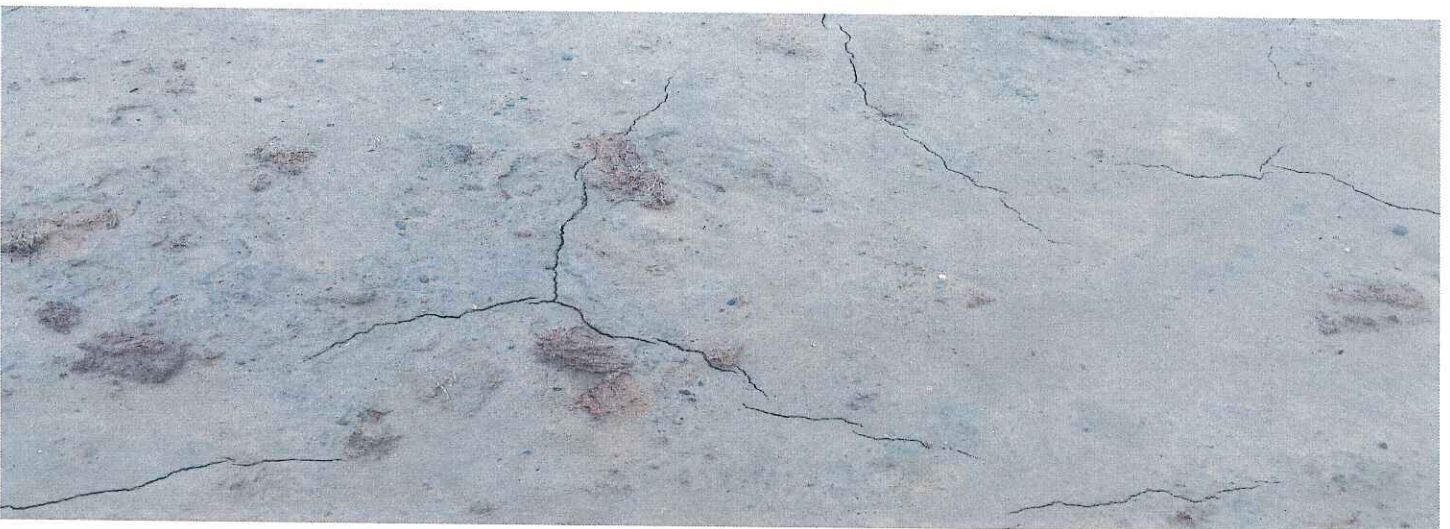
Figure 6 Cracking on new sump cap, July 21, 2020
