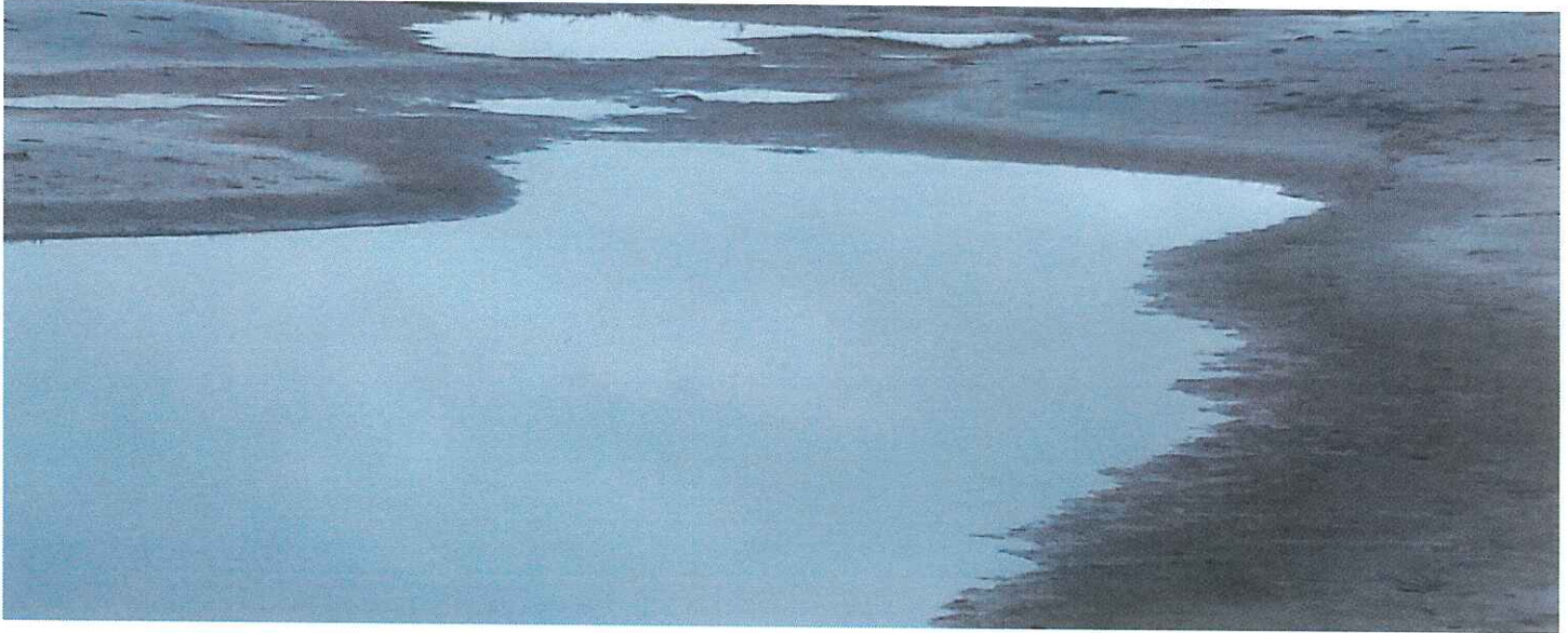
Figure 4 Water Ponding on sump, July 21, 2020
