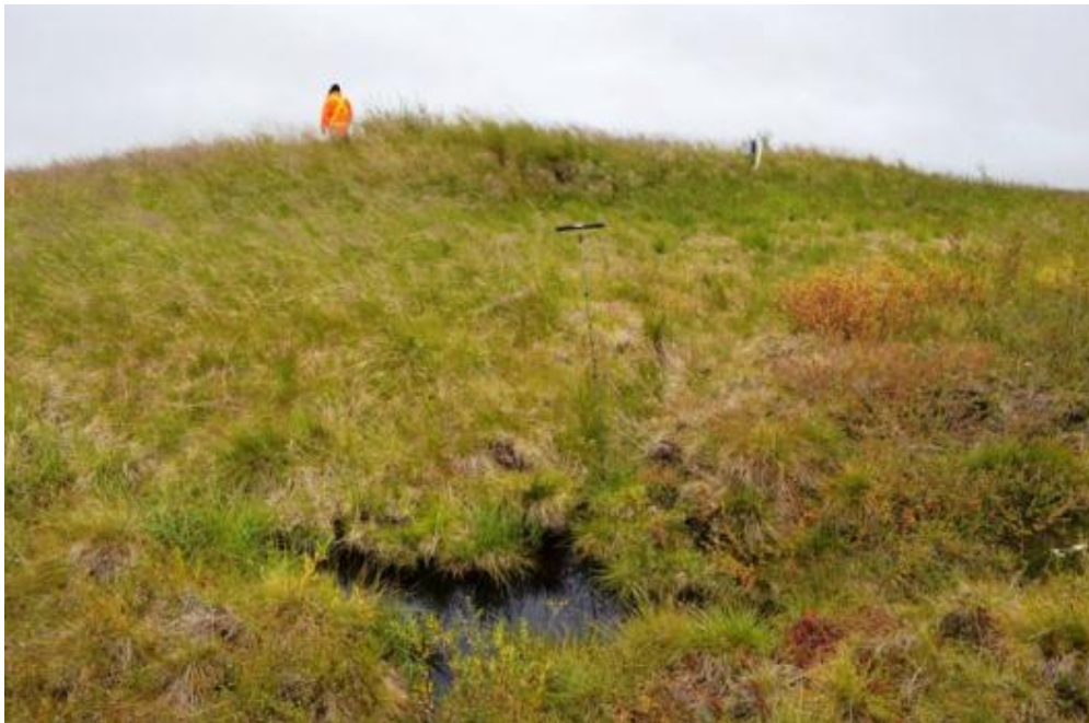
Photo 6 Water ponding at the intersection between two ice-wedges; northwest corner of the sump. August 2015.
