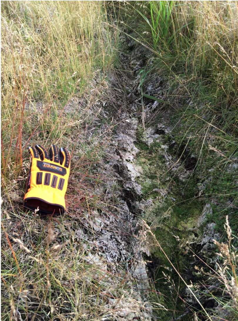
Photo B-3 N-16 Wellsite: View of shallow linear depression (trough) located above a suspected ice wedge near wellhead (looking east). August 22, 2016.
