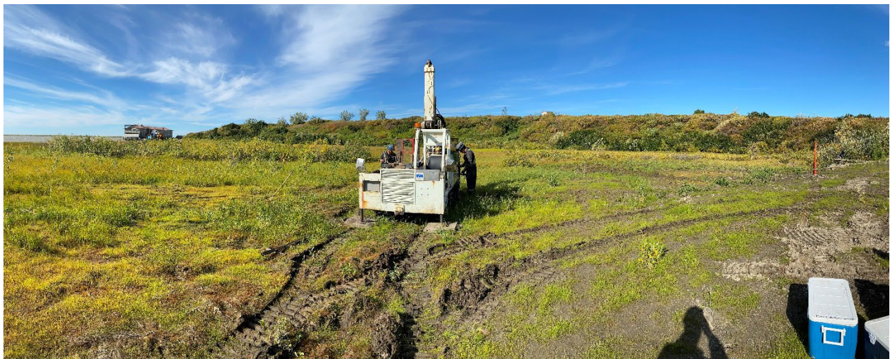
Photo 16 – Drilling BH22-60. The barge camp is visible on the left and MW22-22 on the right, facing northwest (August 26, 2022).
