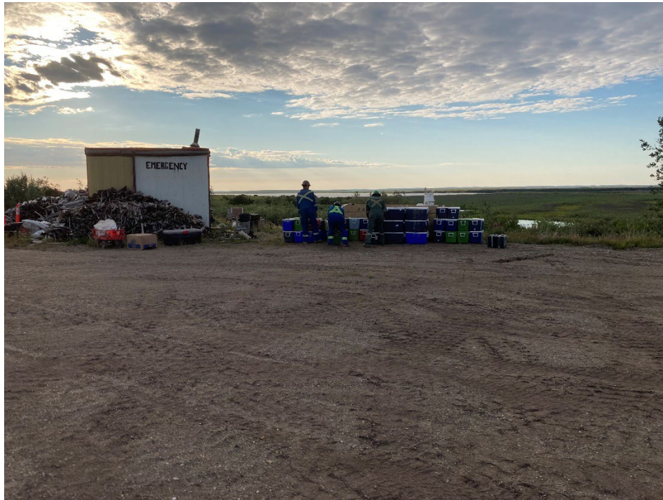
Photo 3 – Preparing the Site for drilling activities. The emergency shack, wood piles, field staff and sample coolers are visible, facing southeast (August 5, 2022).
