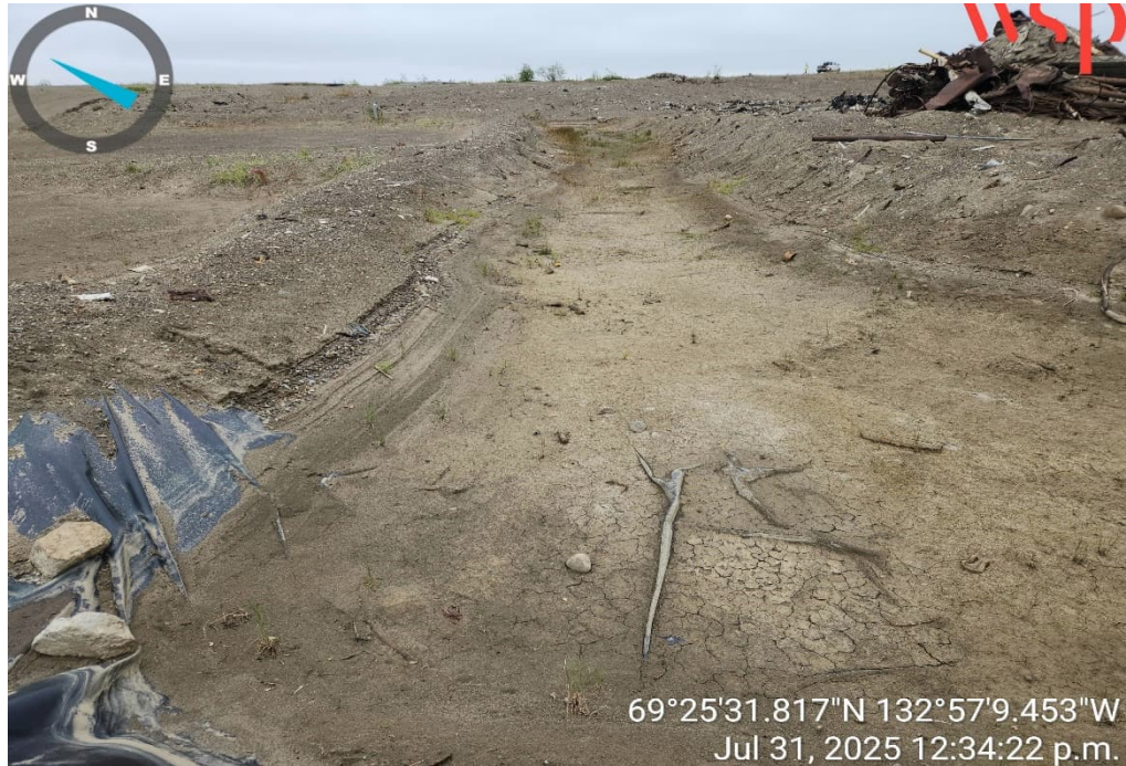
Photo 7 – Sedimentation within swales at Metal & Debris Stockpile (31 July 2025).
