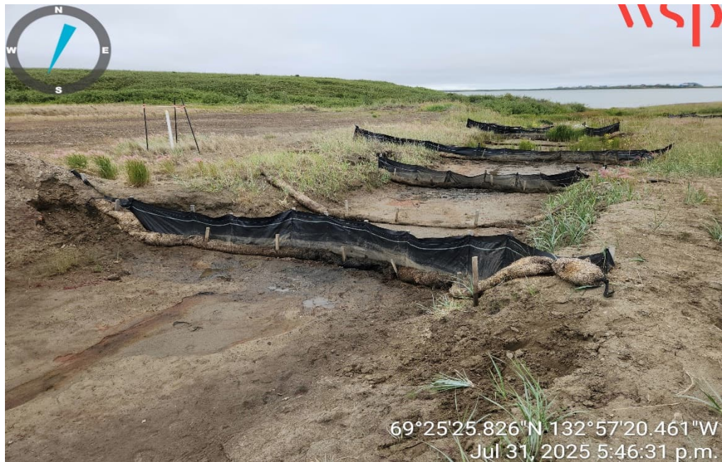
Photo 8 – Repaired silt fence in the Lower Terrace main water management swale (31 July 2025).
