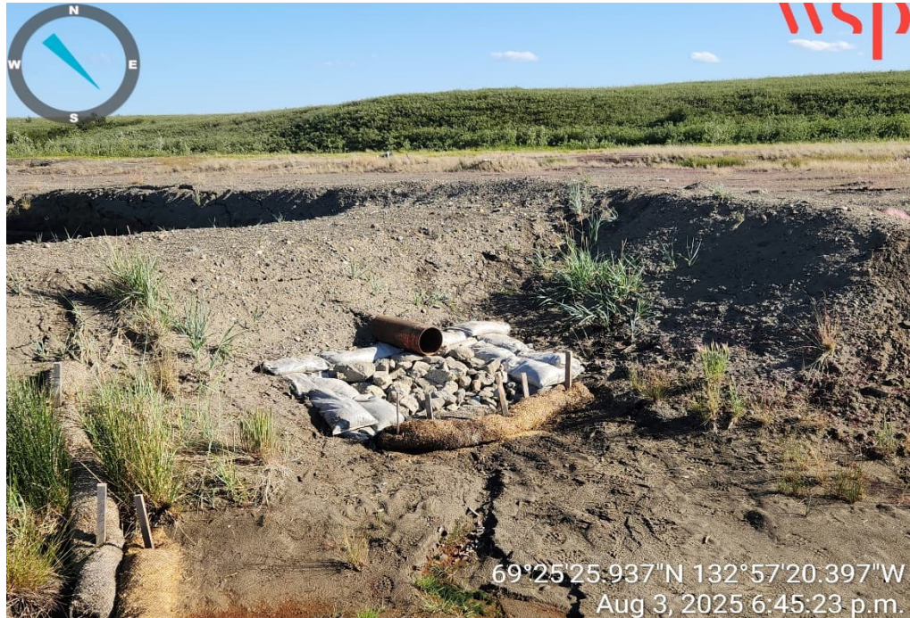
Photo 19 – Additional rip rap added to splash pad of overflow pipe from the main secondary settling pond (3 August 2025).
