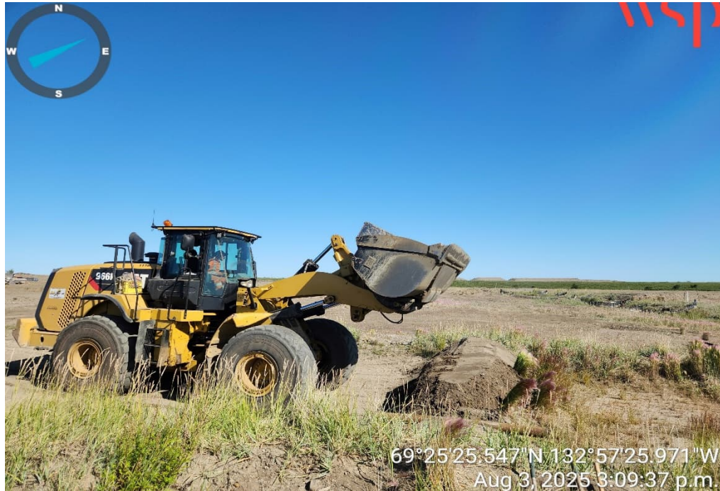
Photo 17 – Rebuilding berm surrounding the southwest settling pond for swales at the Metal & Debris Stockpile (3 August 2025).
