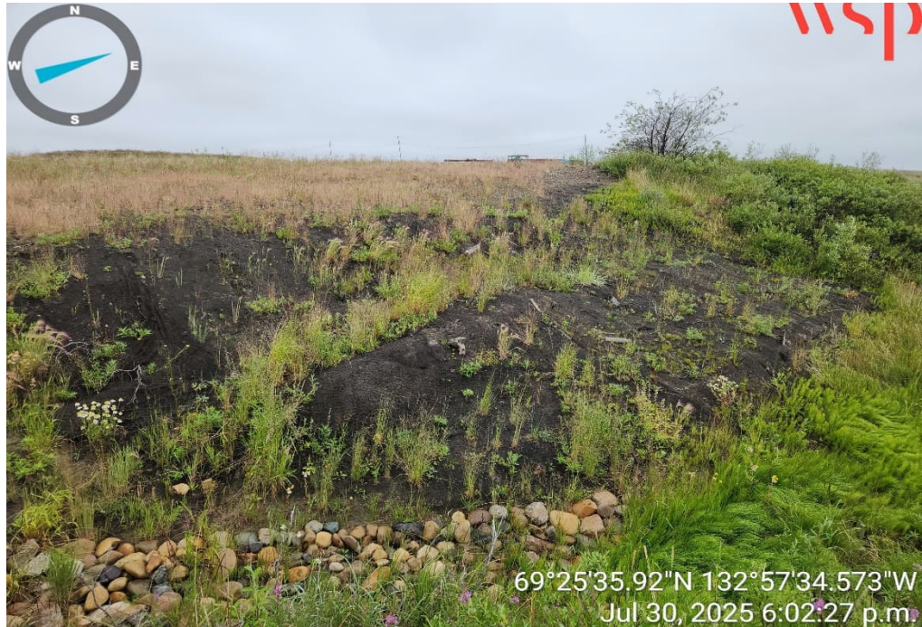
Photo 5 – Slope slumping in area of previously remediated D2 on Upper Terrace (30 July 2025).
