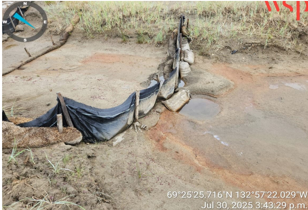
Photo 1 – Sedimentation before repairs were completed at the Lower Terrace main water management swale (30 July 2025).
