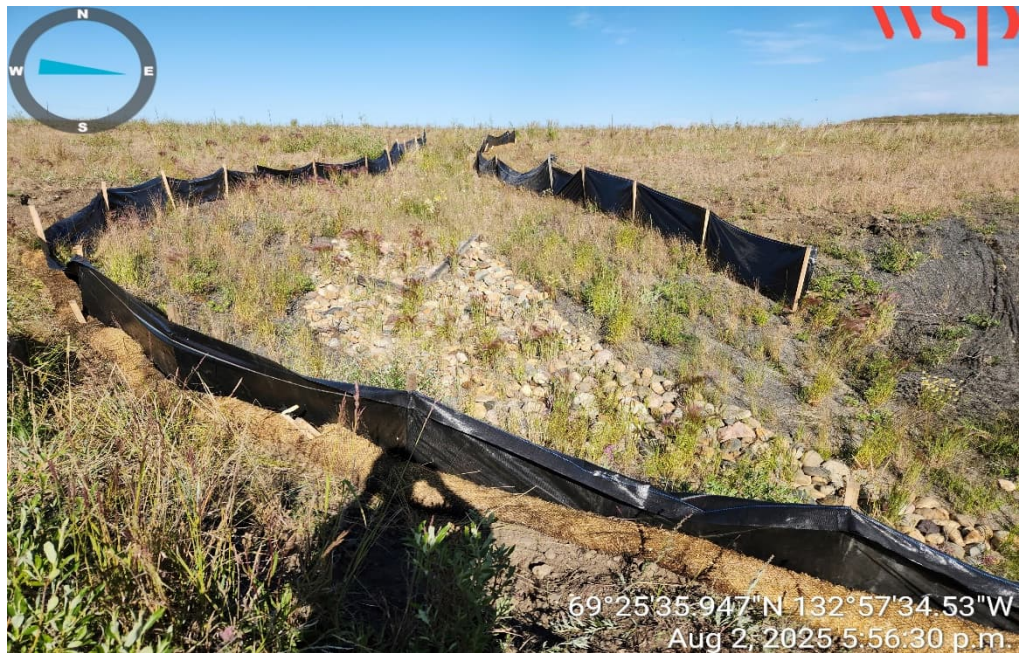
Photo 14 – New silt fence and wattles installed on each side of the ephemeral draw through former remediated excavation D2 (2 August 2025).
