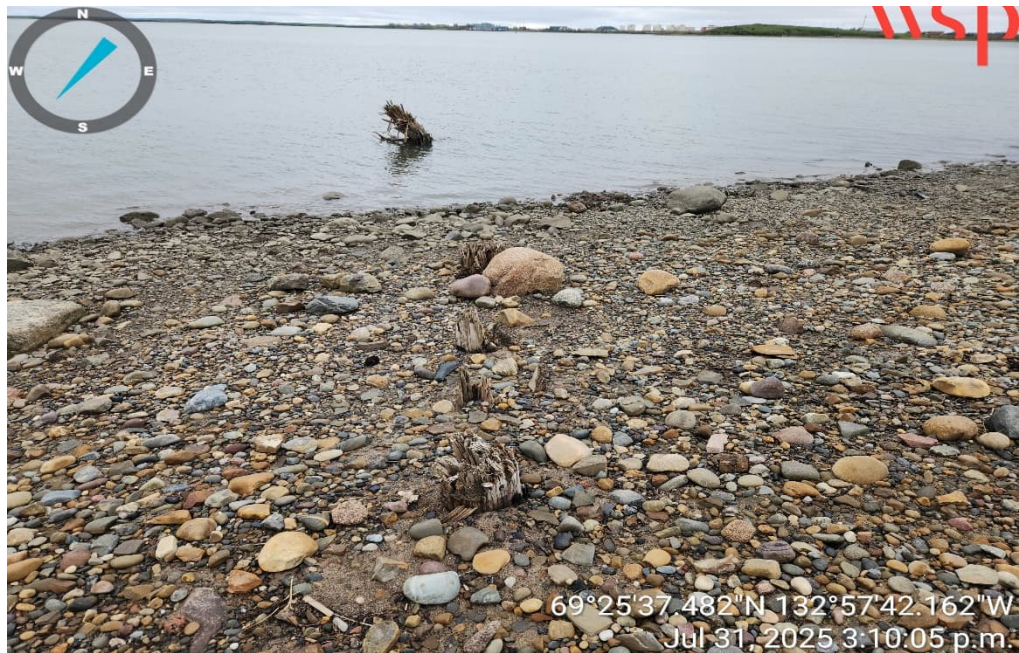
Photo 6 – Exposed wood pilings at the former wood wharf (31 July 2025).
