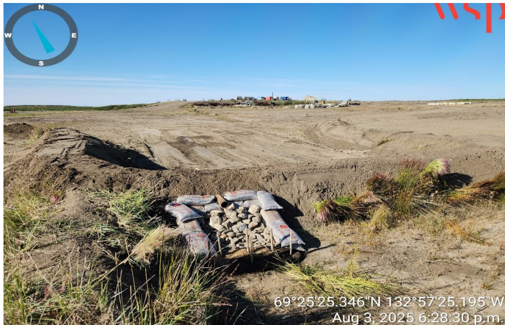
Photo 18 – Completed berm repairs with overflow pipe and splash pad for the southwest settling pond for swales from Metal & Debris Stockpile (3 August 2025).
