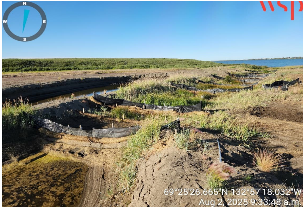
Photo 11 – Completed straw-wattle replacement and minor repairs on the Lower Terrace main water management swale (2 August 2025).
