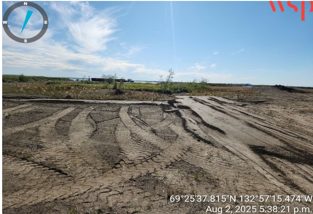
Photo 15 – Repaired soil subsidence on the Upper Terrace adjacent to a former remediated excavation (2 August 2025).
