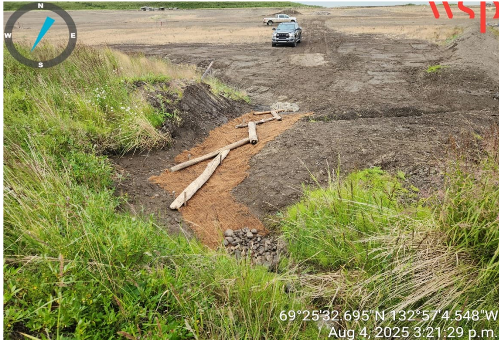
Photo 21 – Constructed erosion control coconut matting and driftwood within the water management swale at the southeast corner outside the South Landfill (4 August 2025).
