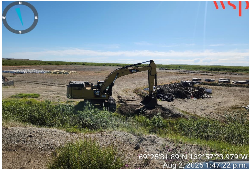
Photo 13 – CAT 349 excavator repairing swales and berms at the north entrance to the Metal & Debris stockpile (2 August 2025).
