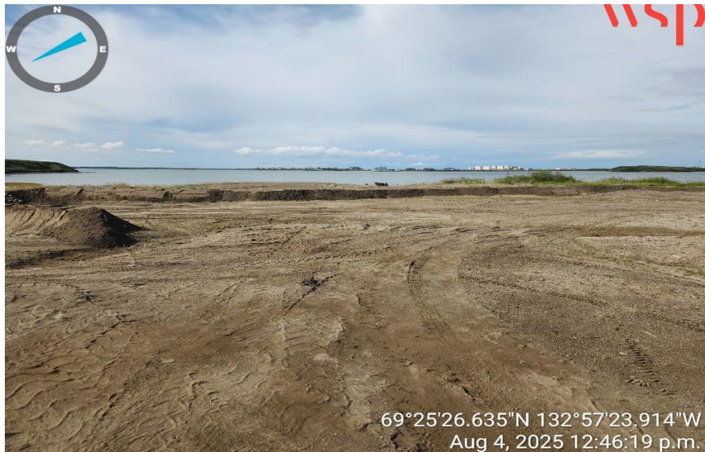
Photo 20 – Extended berm of the southwest settling pond for the swales originating at the Metal & Debris Stockpile (4 August 2025).
