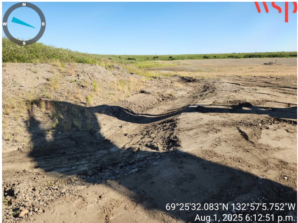
Photo 10 – Restored water management swale at the southeast corner of the South Landfill (1 August 2025).
