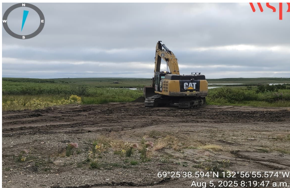
Photo 22 – Backfilled and graded to natural ground elevation at the Former Sewage Lagoon (5 August 2025).
