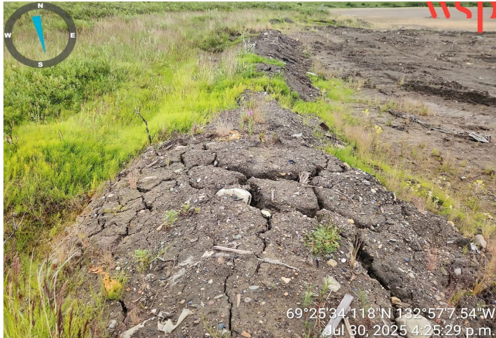
Photo 3 – Berm deterioration around the South Landfill (30 July 2025).
