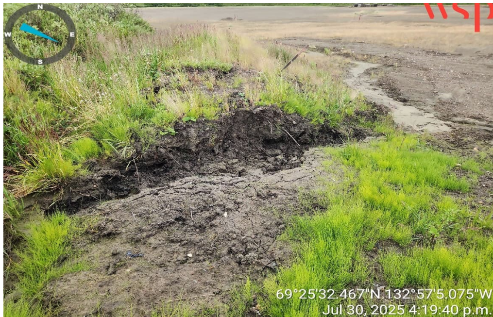
Photo 2 – Erosion from a swale requiring redirection along the east side of the South Landfill (30 July 2025).
