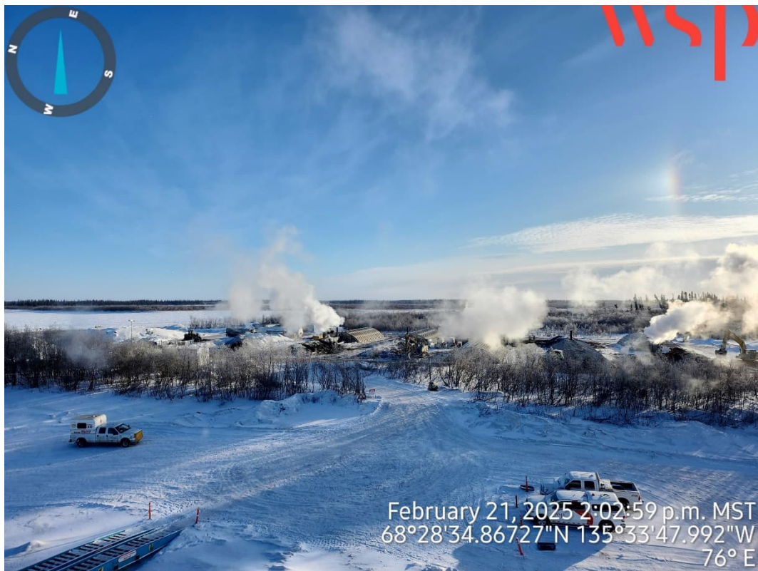
Photo 2 – Site remediation activities, taken from the deck of the barge camp (21 February 2025).
