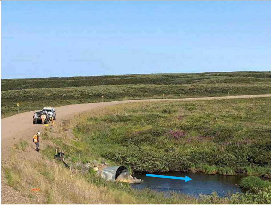
Looking north (Towards Tuk) at the downstream culvert end outlet Note the culvert end is uplifted. Scour pool downstream. Culvert is under sized Photo taken July 25, 2019.
