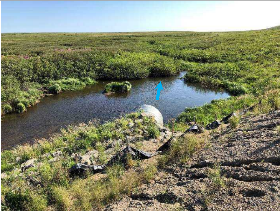
Looking East (Downstream) Note scour pool/ponding and class 1 rock. Existing 2000 mm culvert is undersized Channel is not well defined. Photo taken July 25, 2019.
