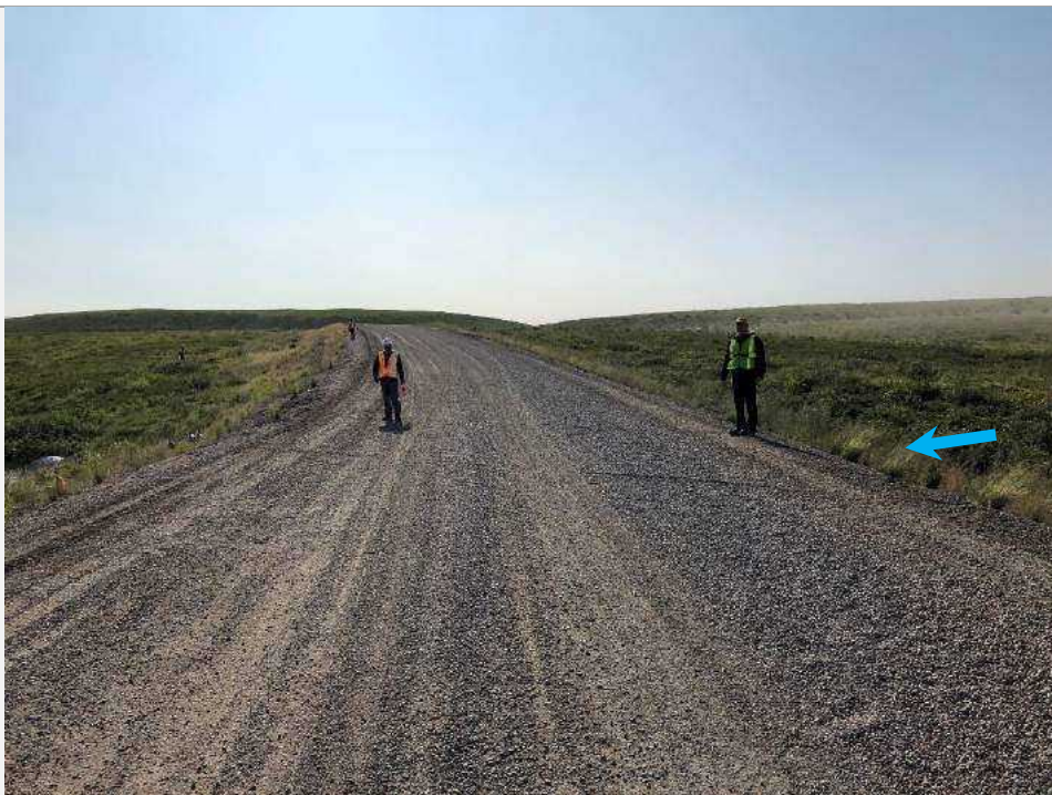
Looking South (Towards Inuvik) along ITH at Gunghi Creek Crossing, Existing 2000 mm SPCSP culvert is at 40 degree RHF skew with roadway CL at Station 131.2. Persons are standing along culvert orientation. Photo taken July 25, 2019.
