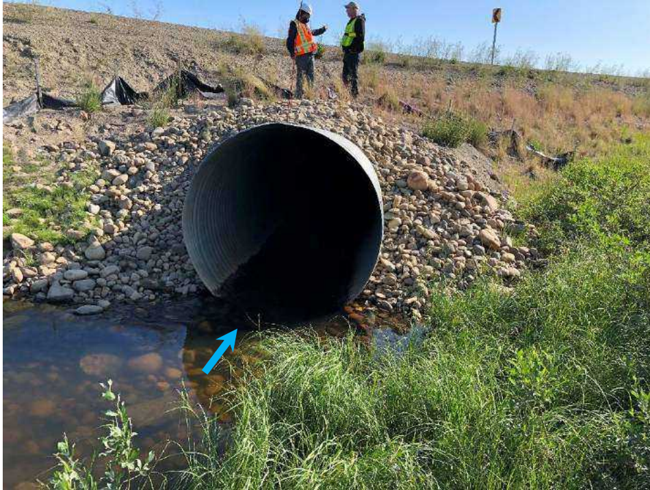
Looking east (upstream culvert end) Note class 1M rock. Photo taken July 25, 2019.
