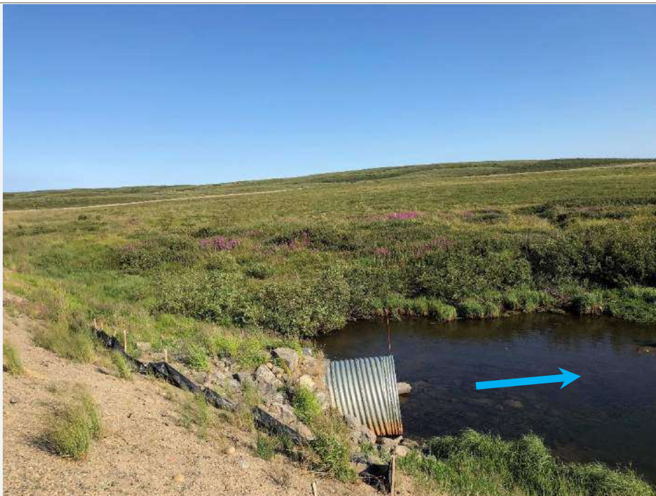
Looking north at the downstream culvert end outlet Note the culvert end is uplifted. Photo taken July 25, 2019.
