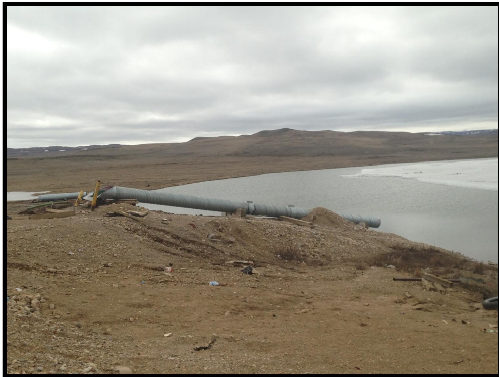
Figure 11: Sewage Disposal Facilities Discharge Chute
