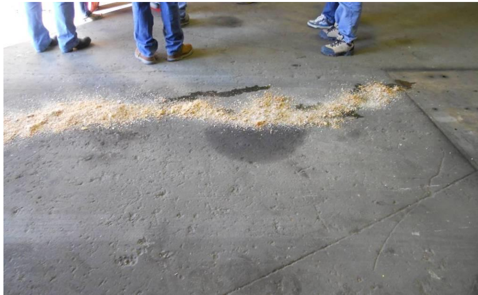
Figure 4: Absorbent Material Placed over Spilled Vehicle Fluids
